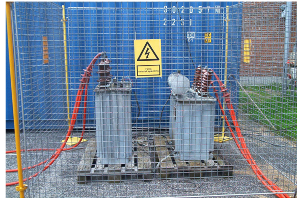
Fig.3.4. Photo of high voltage transformers used to generate 10-kV system.
