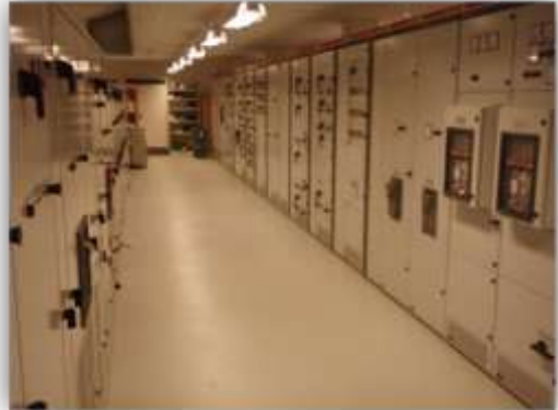
Part of the switch room
