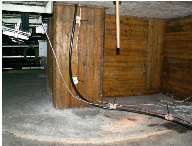
fig. 65. Photo of Cable1 in parallel to GroundWire1
