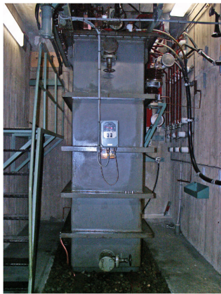
fig. 63. Photo of transformer T2
