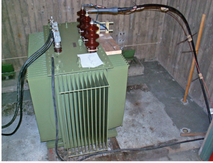
fig. 68. Photo of Transformer TX2
