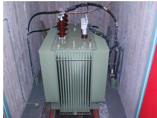
fig. 64. Photo of transformer TX1
