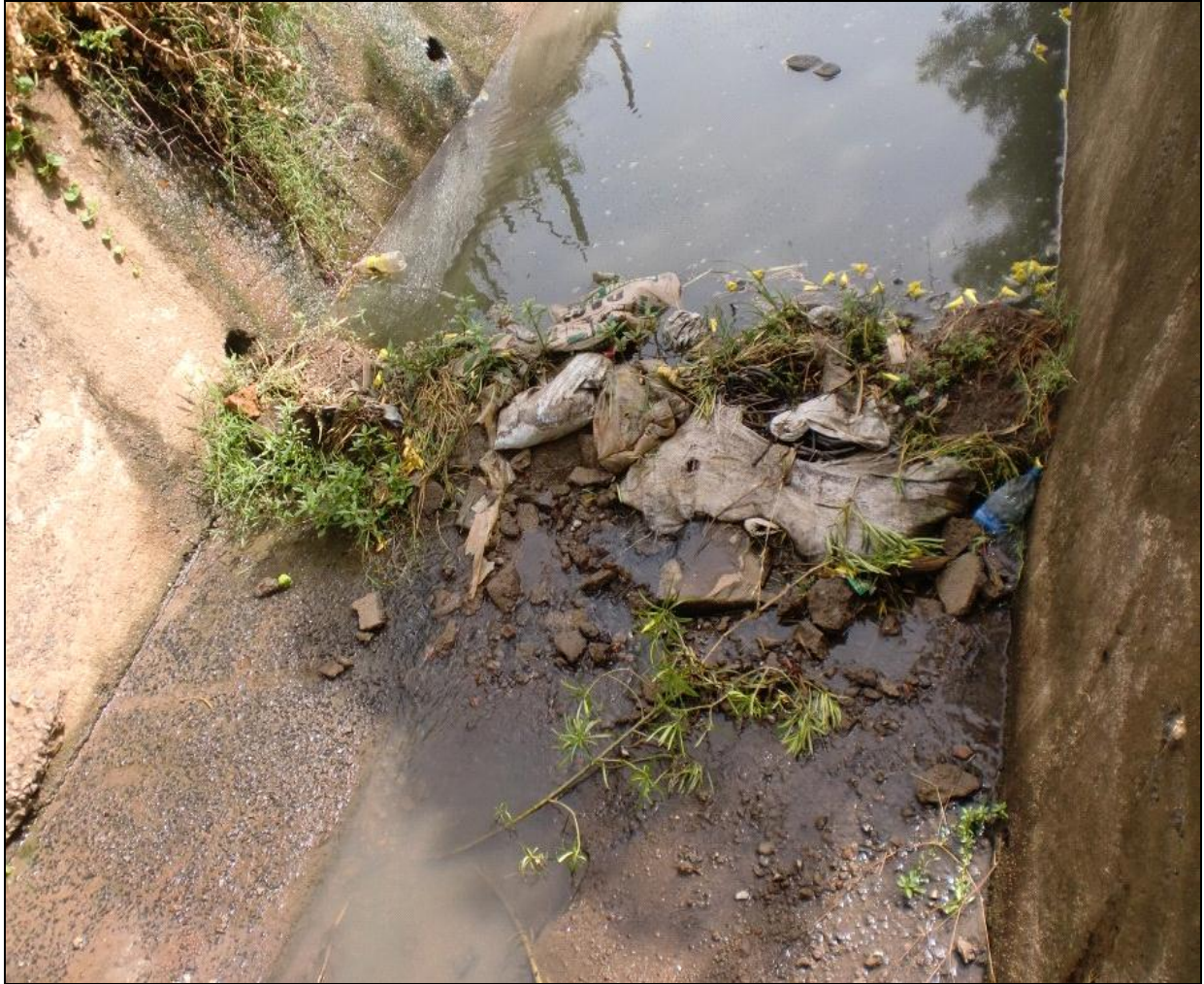
Plate 8. A picture showing a clogged drain at Carwash
