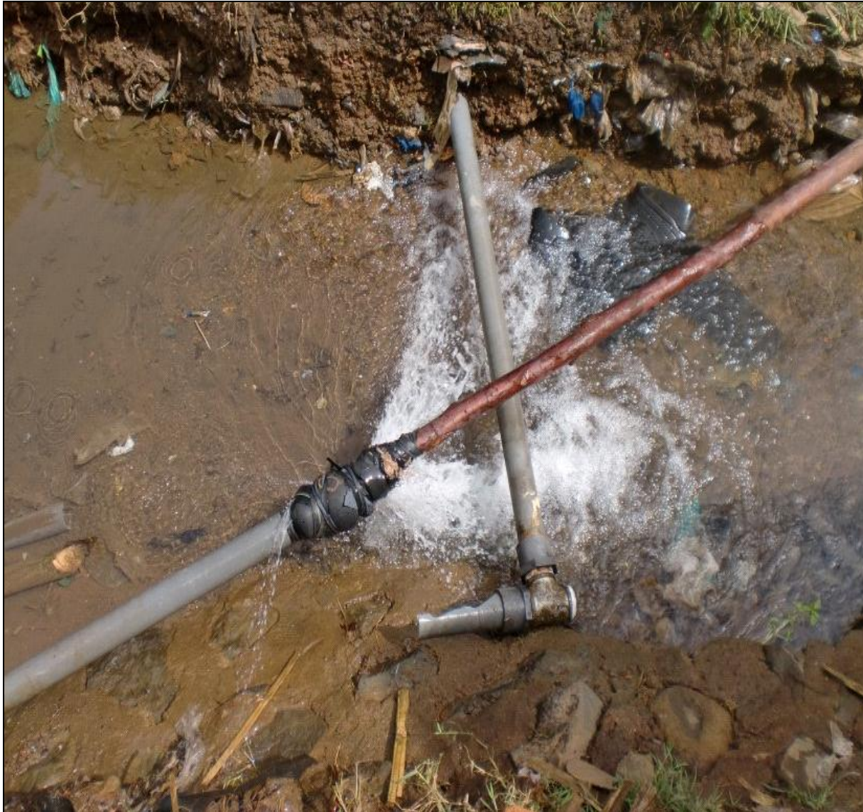
Plate6. Picture showing a broken pipe at Carwash, contamination points
