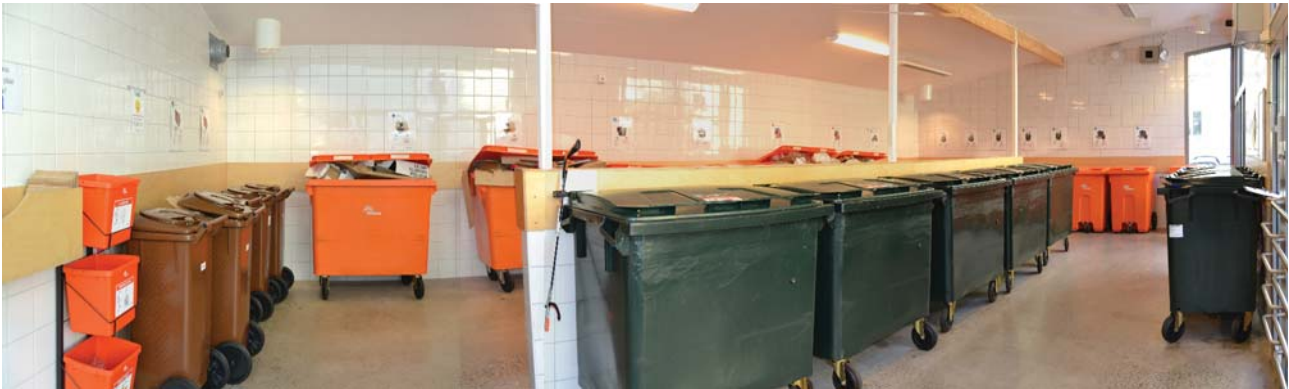
Figure 15: Waste sorting room located in the city centre that participated in case study B. This room tested the sealable bags maintaining the lid on the bio-waste containers (brown containers seen at the right side of the picture).
